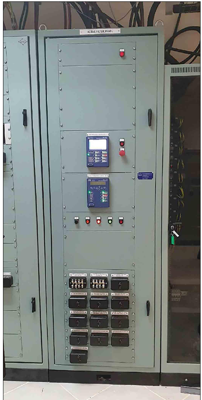
Figure 2: New protection and control panel implemented
