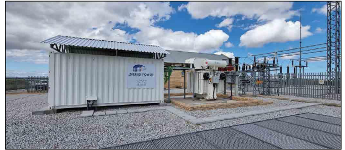
Figure 5: Active harmonic filter and step-up transformer installation
